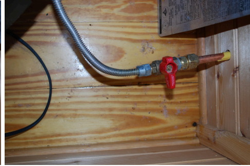
GAS OFF POSITION
